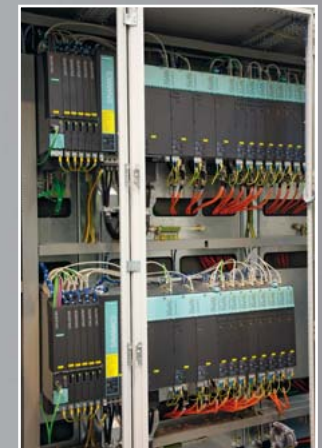
■ Drive control unit SIEMENS
